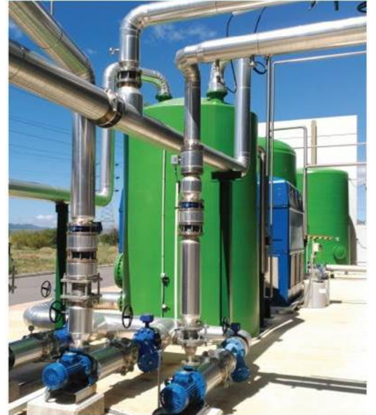
CLAMBER Pilot Plant
